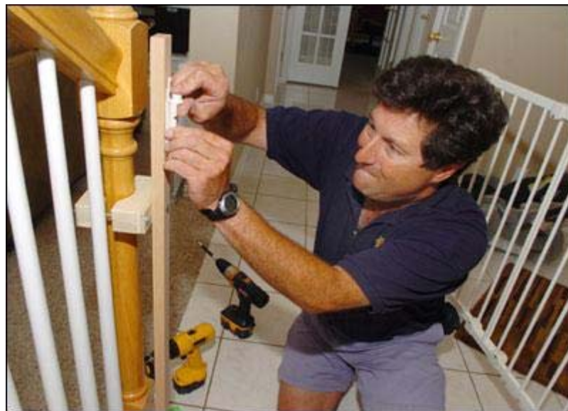
Lou Delaware, owner of Colorado Childproofers, installs a staircase gate in a house in Lafayette, using techniques that don't damage the rails and posts. (Post / John Epperson)
